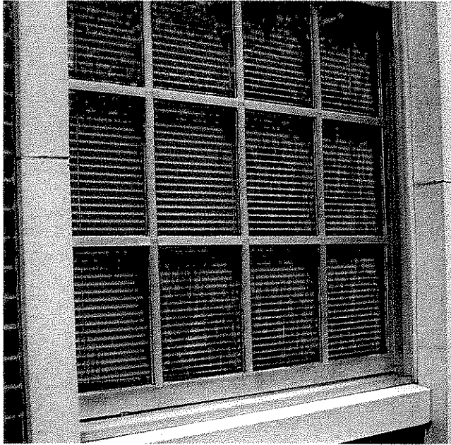
Note condensation in window frame
